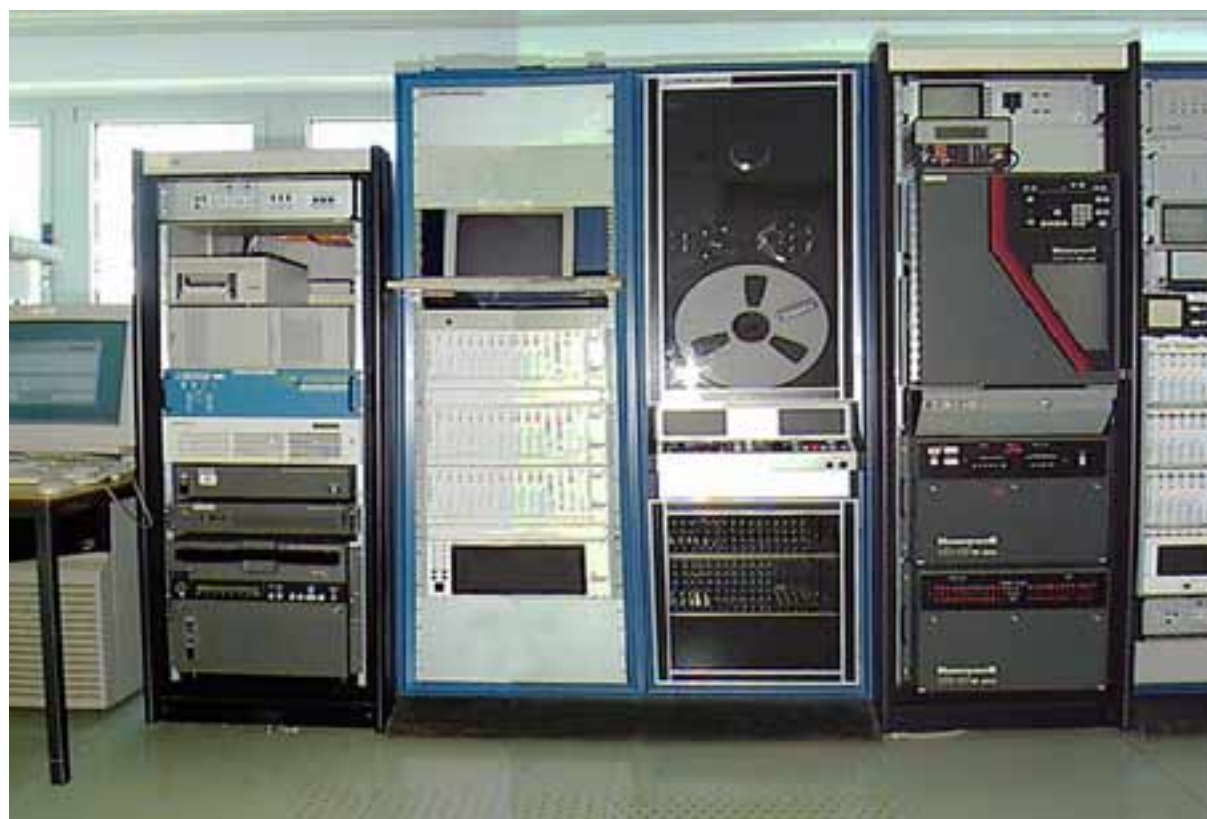
Figure 6: Three generations of storage devices at D-PAF.
